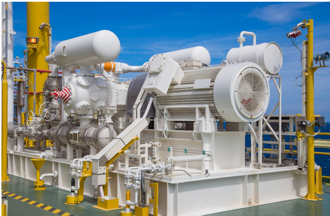
High pressure gas compression on an offshore rig
